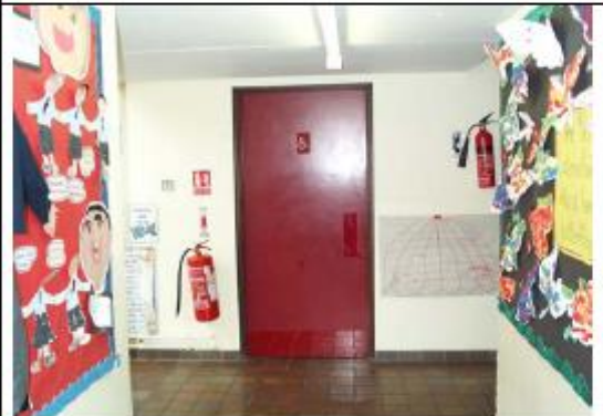
Photograph 4 Poor contrast of colour on the accessible WC door.
